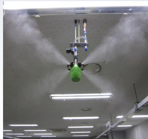
Automatic Humidity Control System
